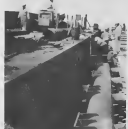
Above, progress is underway on a job required for the turnaround of the West Pier at Arriba, involving the driving of steel piles under the existing structure of the walkway for the construction of a completely new fendering system.
